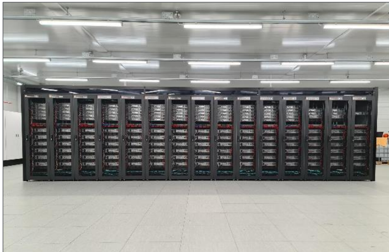
DestinE Data Bridge Infrastructure in LUMI
