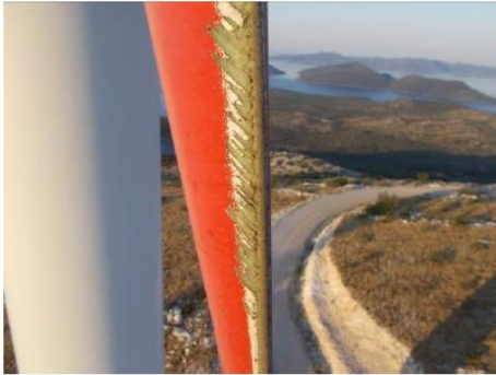
Photo 1: Erosion LE. Z33 and 35,2m
