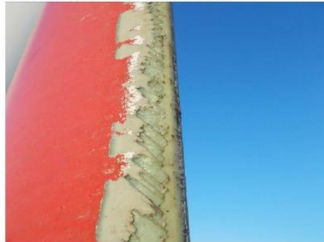
Photo 4: Erosion LE. Z33 and 35,2m
