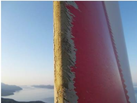
Photo 5: Erosion LE. Z33 and 35,2m
