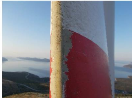
Photo 6: Erosion LE. Z33 and 35,2m
