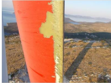
Photo 2: Erosion LE. Z33 and 35,2m
