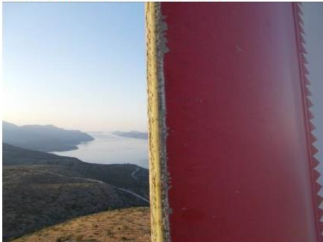
Photo 3: Erosion LE. Z33 and 35,2m
